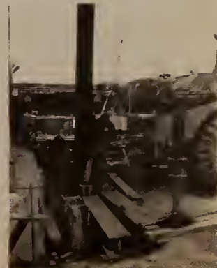
Production pile being placed near Casey Highway pier as support for underpinning.
